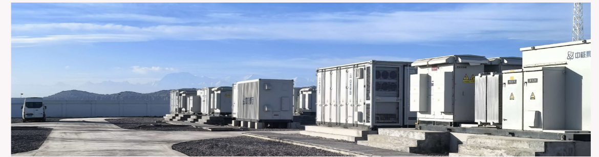
■ 80MW/160MWh Grid-forming Energy Storage Project in Shufu County, Kashgar, Xinjiang
