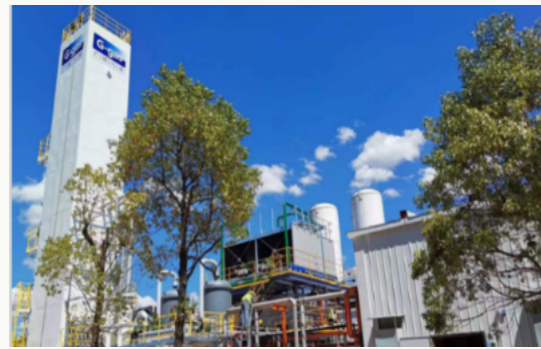
Energy-Saving Technological Transformation of On-Site Nitrogen Generation
